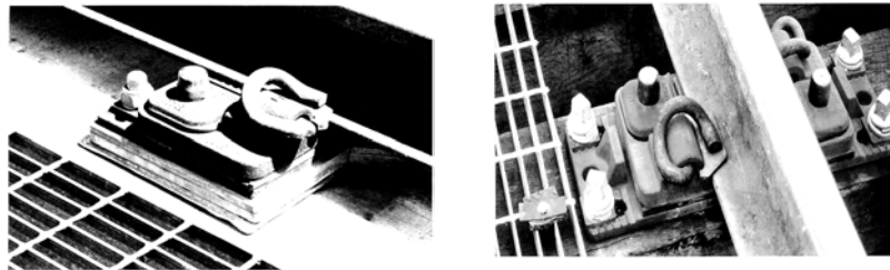
Fig. 1 – Elastic systems for fixing the railway lines.
