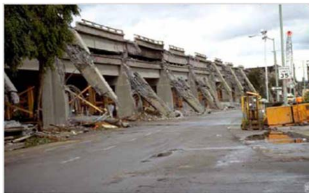
Fig. 2 – Cypress Viaduct - Loma Prieta earthquake, 1989.
